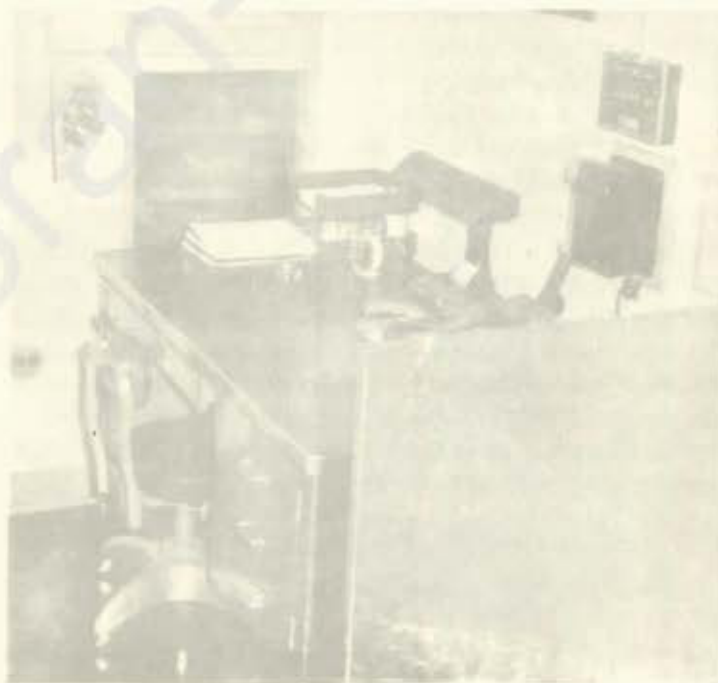
Office Note automatic fire alarm system zone indicating panel on wall
