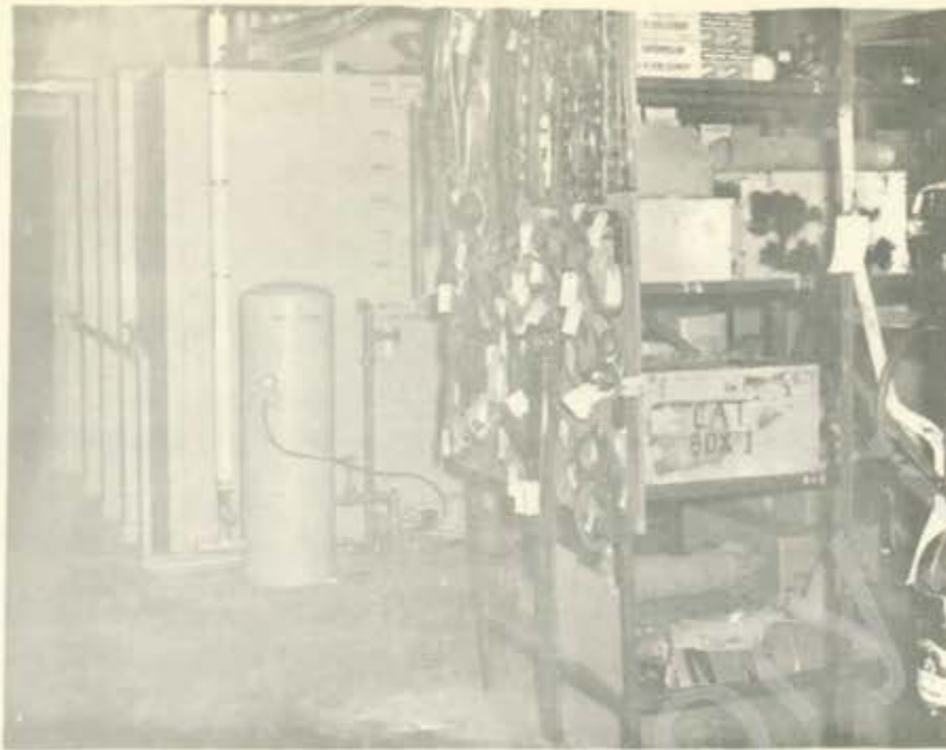
Engineer's Storeroom In Power Building #2 The #2 fresh water tank and #2 domestic fresh water pump can be seen. Looking toward tank room #2.
