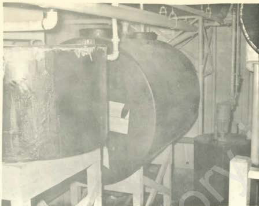
Sewage Tank Room...Tanks: (l. to r.) Syphon, Septic And Waste Water Accumulator. Looking toward Crew's Bath Room.
