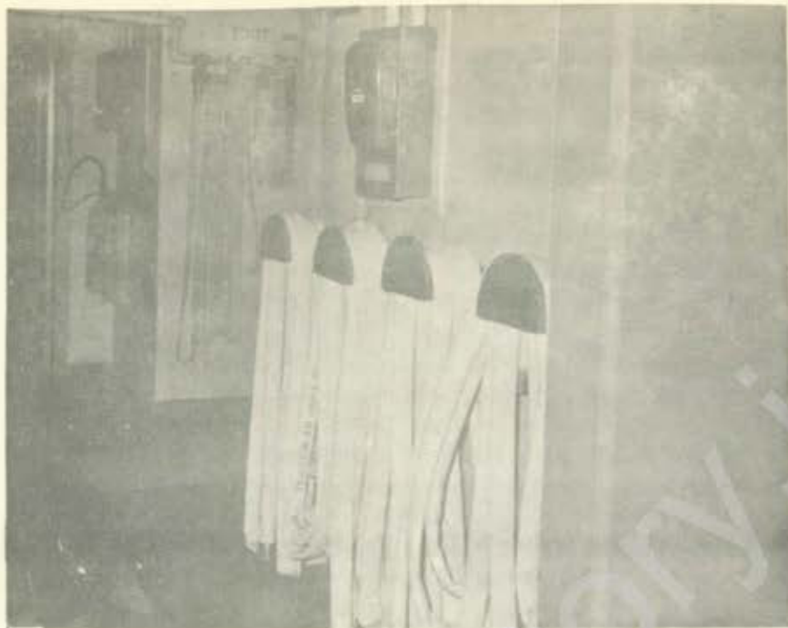
Central Passageway Showing Fire Fighting Equipment
