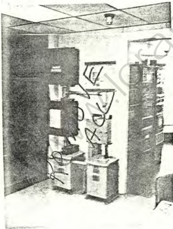
Isolation transformers and line filters used with AN/FPN-30 timer and AN/FPA-2 switchgear. No longer required, scheduled for removal.
