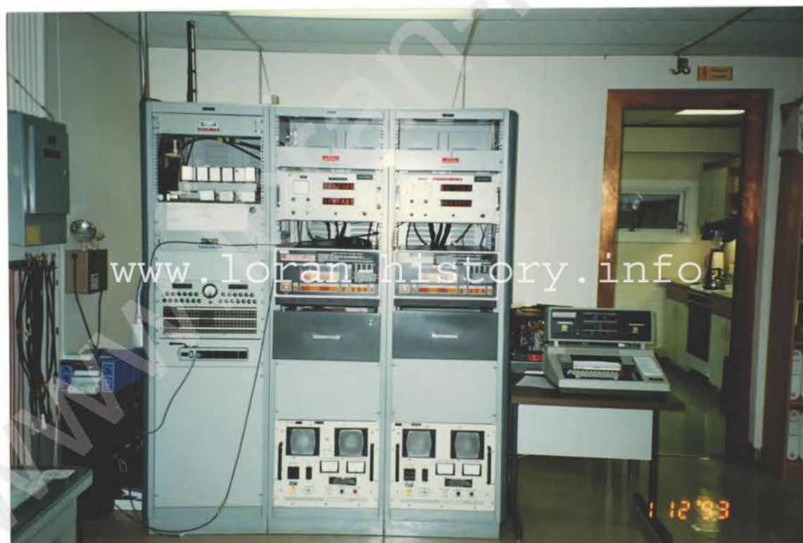
SOME LORAN MONITOR EQUIPMENT LOCATED IN STATION OFFICE SPACE
